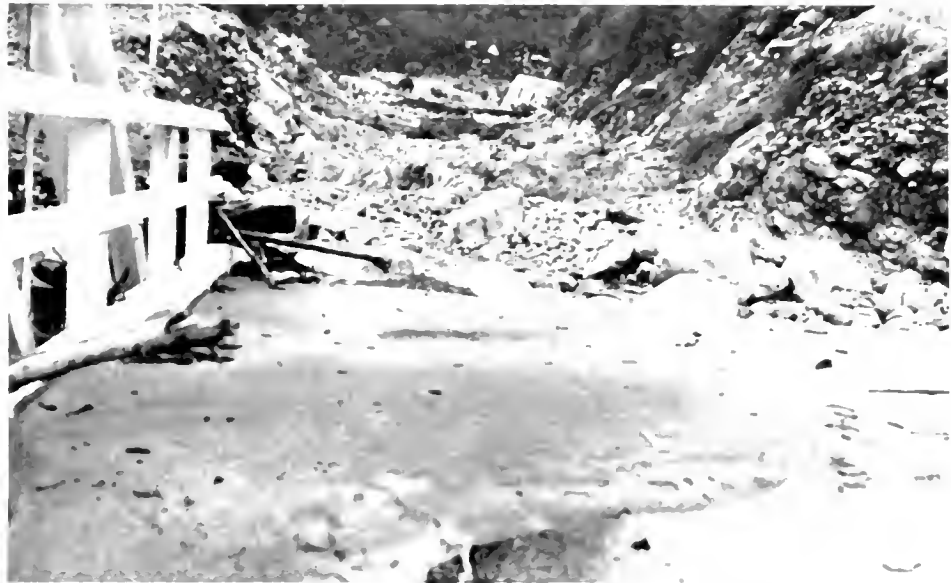
Roadway between bridges washed out in San Gabriel Canyon
